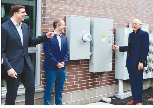
Rep. Adrian Madaro (left) and Dan Lesser, Chief of Staff to Sheila Dillon, Mayor's Office of Housing, joke with NOAH's Executive Director, Phil Giffie (right) as he turns on the solar power at Coppersmith Village.
